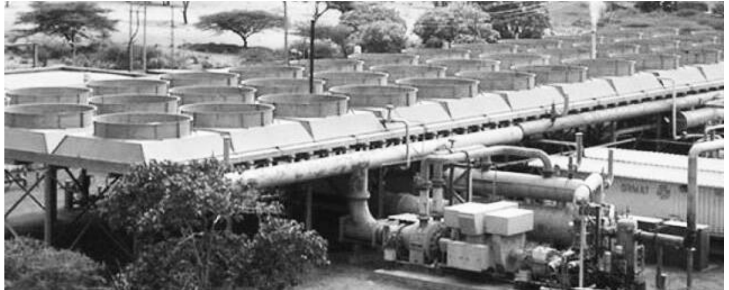
Ethiopia's Aluto Langano Geothermal Project operational
