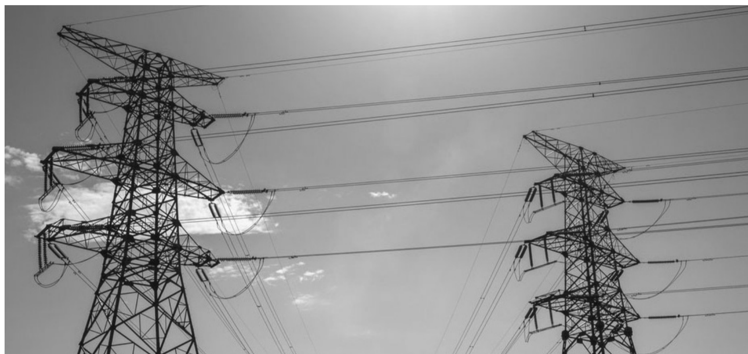
Some of the electric transmission lines
