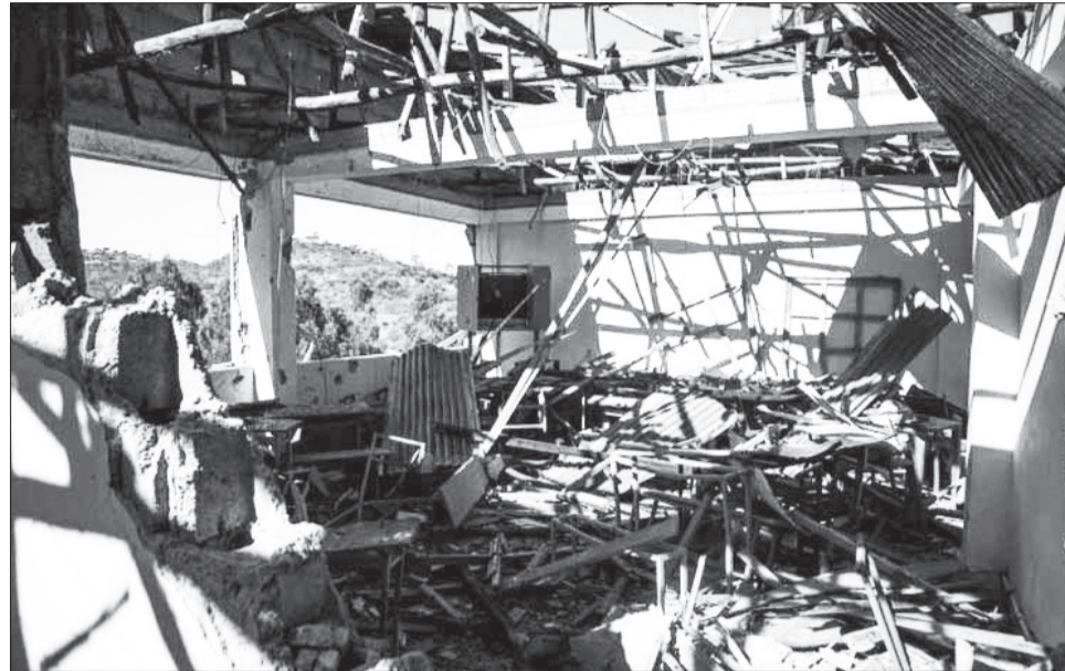
T-TPLF destroyed 832 schools in North Wollo, in the regional state of Amhara
